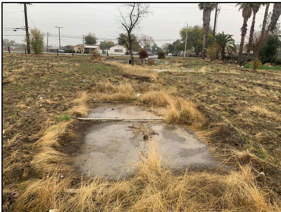
Plate 3.2-19: Overview of the concrete pads, facing east. The western-most concrete pad is in the foreground and the central concrete pad is in the background, in front of the foundation.
